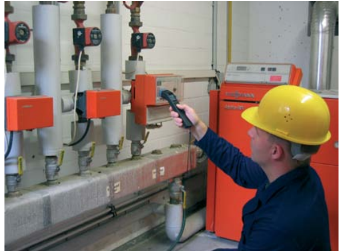
Checking the temperature of heating circles
